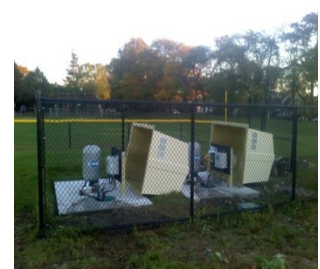
Artesian Well Submersible Pump System, VFD Drive System, Tank System & Water Filtration System
