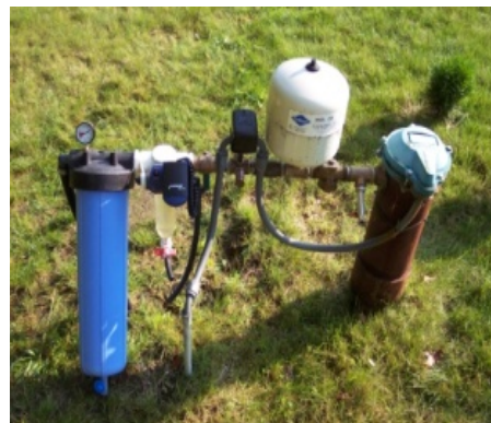
1 micron bag filter for removal of fine sand and silt from irrigation well (Hopkinton, MA)
