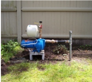
Shallow Well Jet Pump System & Tank System
