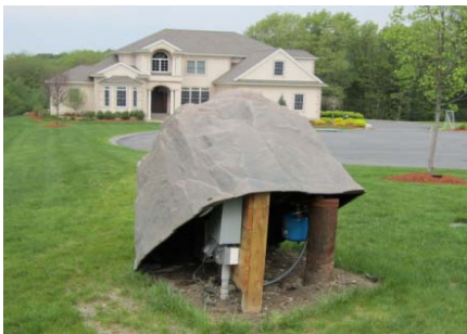
Well , Tank & Electrical components hidden under Artificial Rock Wayland, MA
