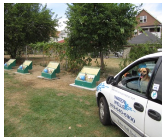
Four (4) Point Well Systems enclosed in insulated enclosures Belmont, MA
