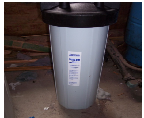
Cartridge Filter to remove sediment from well in whole house water system (Stoughton, MA)
