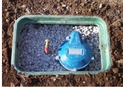
Well-head Cut Below Grade and installed in jumbo irrigation box with cover Wilmington, MA
