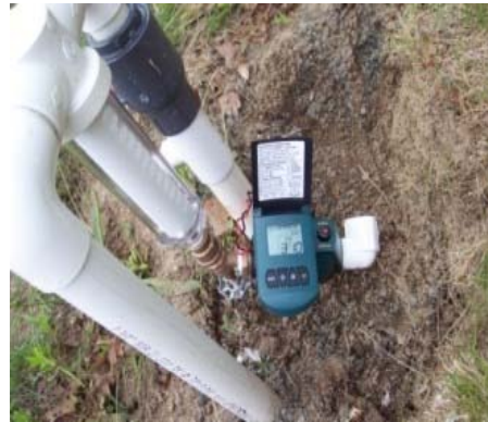
Clear View sediment filter including "Automatic" flush valve for irrigation well (Canton, MA)
