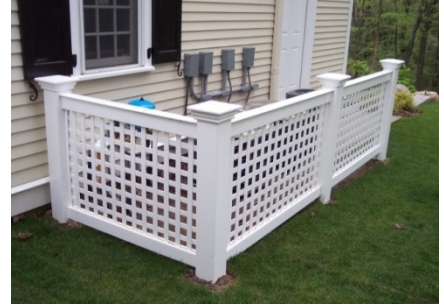
Screen custom-built on site for homeowner to hide Constant Pressure System Concord, MA
