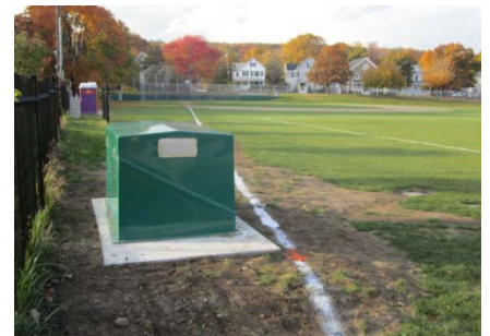
5 hp 50 gpm Pumping System installed in insulated enclosure Belmont, MA
