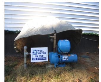
Point Well and pump system hidden under Artificial Rock Tewksbury, MA
