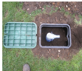
Point Well installed in large irrigation box with cover N. Reading, MA
