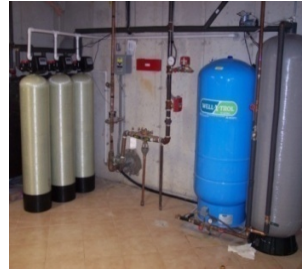
Artesian Well Submersible Pump System, Tank System & Water Treatment System
