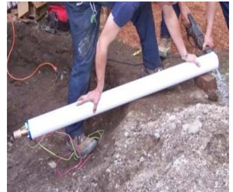
Pump Screen installed over submersible pump to limit intake of sediment from irrigation well (Wilmington, MA)
