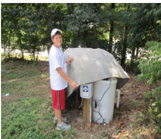
Well, Pump, Sediment Filter & Iron Stain Prevention System under Artificial Rock Braintree, MA
