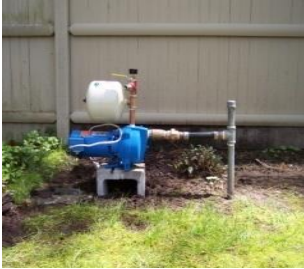
Shallow Well Jet Pump System & Tank System
