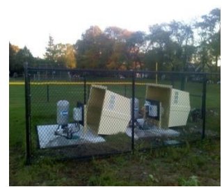
Artesian Well Submersible Pump System, VFD Drive System, Tank System & Water Filtration System
