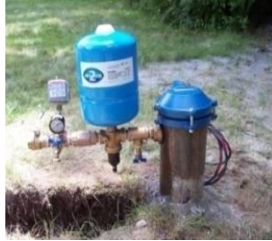
Artesian Well Submersible Pump System & Mechanical Constant Pressure System
