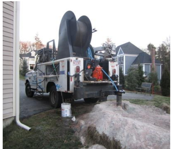
A pump test is performed afterwards to determine the new flow rate (North Reading, MA)
