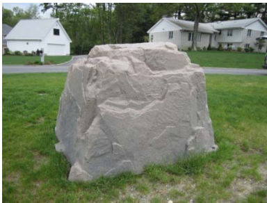
Well , Tank & Electrical components hidden under “Artificial Rock”.
