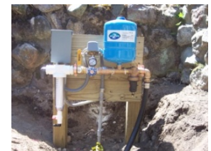
Constant Pressure System and controls mounted outside on pressure treated lumber. (Dedham, MA)
