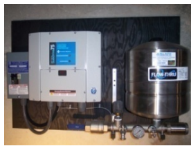
Variable Drive Constant Pressure System with stainless steel tank components and NEMA 4 controller. Mounted on board. (Tewksbury, MA)
