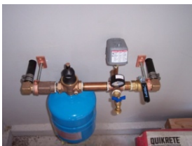
Constant Pressure System for sprinkler system mounted inside garage. (Wayland, MA)
