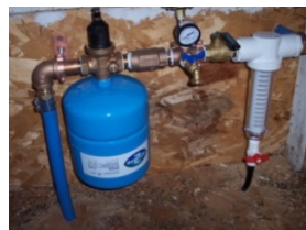
Constant Pressure System including filter and electrical components mounted in shed. (Wilmington, MA)
