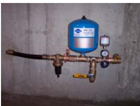
Constant Pressure System mounted in basement of home with additional port for future expansion. (North Reading, MA)
