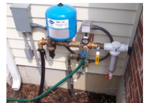
Constant Pressure System on side of house with electrical components and sediment filter. (Milton, MA)
