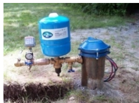
Constant Pressure System mounted to well, for hoses to garden, sprinklers and pool. (Franklin, MA)
